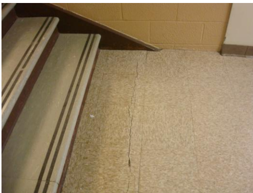
CRACKED FLOOR TILE
