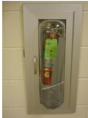
BROKEN FIRE EXTINGUISHER COVER
