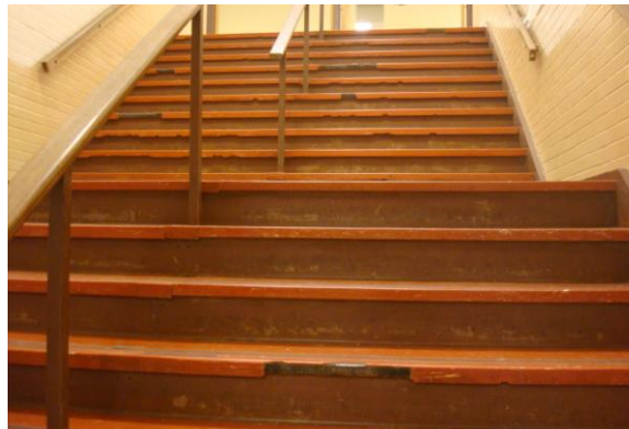
STAIRS WITH CRACKED TREADS
