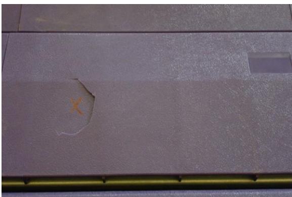
CRACKED BLEACHER FACE
