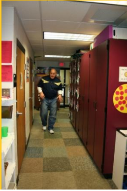
LACK OF SEPARATION BETWEEN KINDERGARTEN CLASSROOMS
