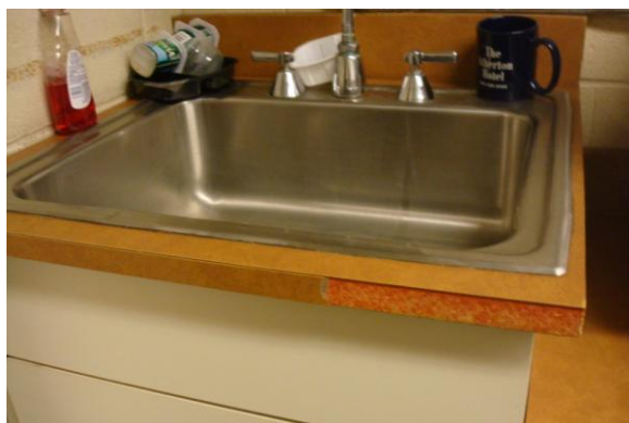
SINK WITH DELAMINATED EDGE
