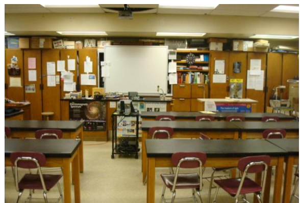
SCIENCE LAB WITH HUMIDITY SAGGED CEILING TILE (roof above has been repaired)
