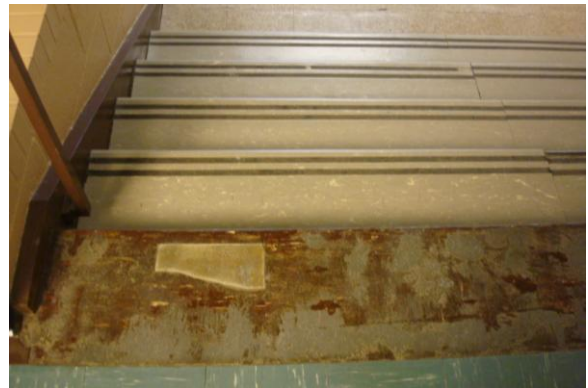
MISSING TILE AT STAIRS
